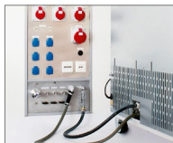
Direct connection to ultrapure water pressure line
